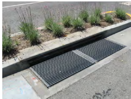
New catch basins were installed as part of the Santa Monica Boulevard Reconstruction Project.
