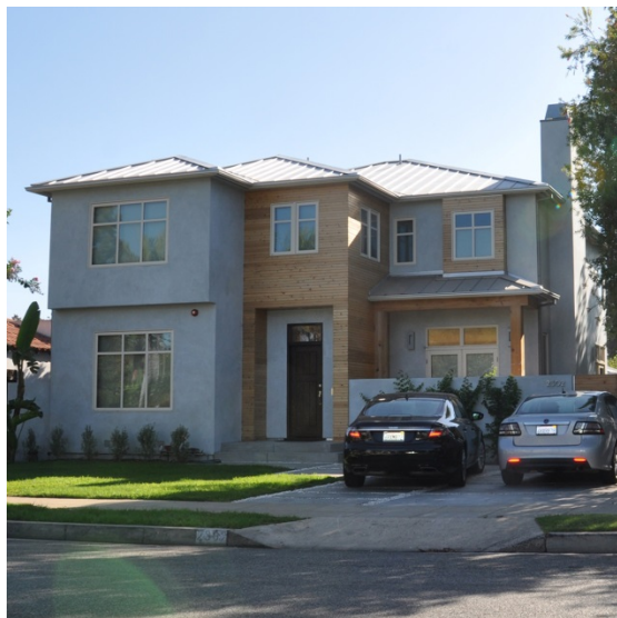
⊗ The windows are of poor quality, finishes do not enhance building design.
