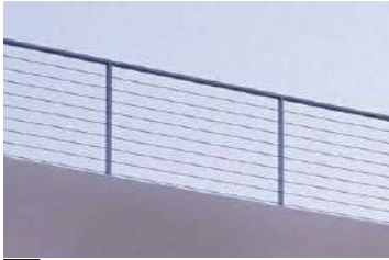
15 FALL PROTECTION RAILING
