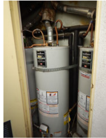
14. View of tenant water heaters at subject property
