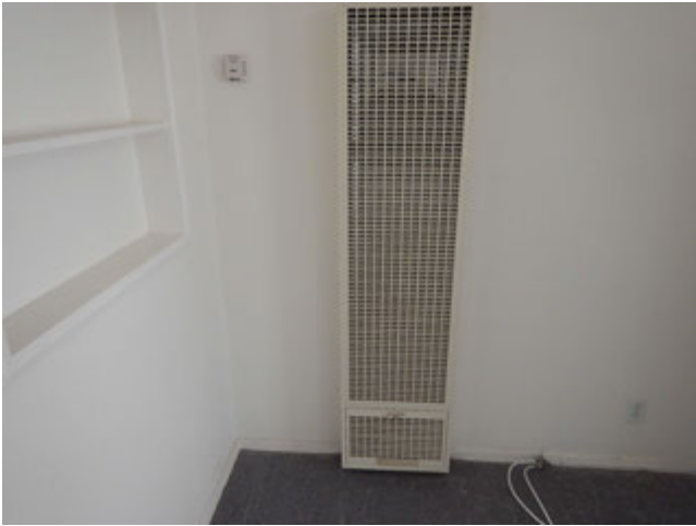
13. View of typical wall furnace at subject property
