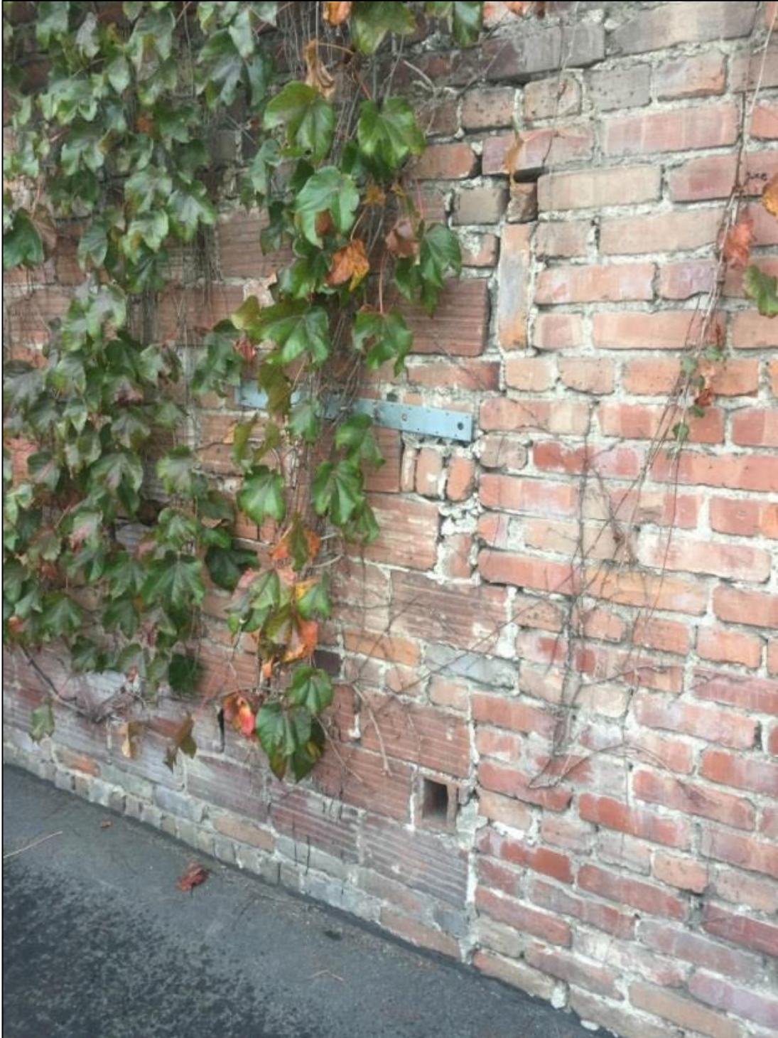
Figure 12. Detail of north elevation, showing the brick and hollow clay tile wall components.
