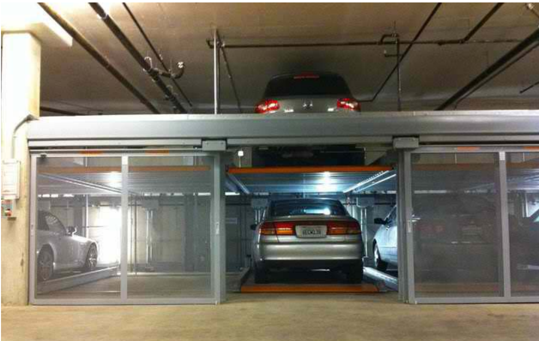
Figure 3 Example of a two-level dependent mechanical lift system, which may require a valet operator.
