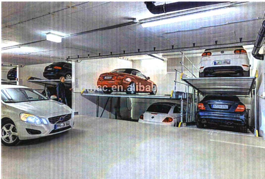
Figure 2 Example of a two-level independent mechanical lift system, where driver can access vehicle without moving the vehicle below.
