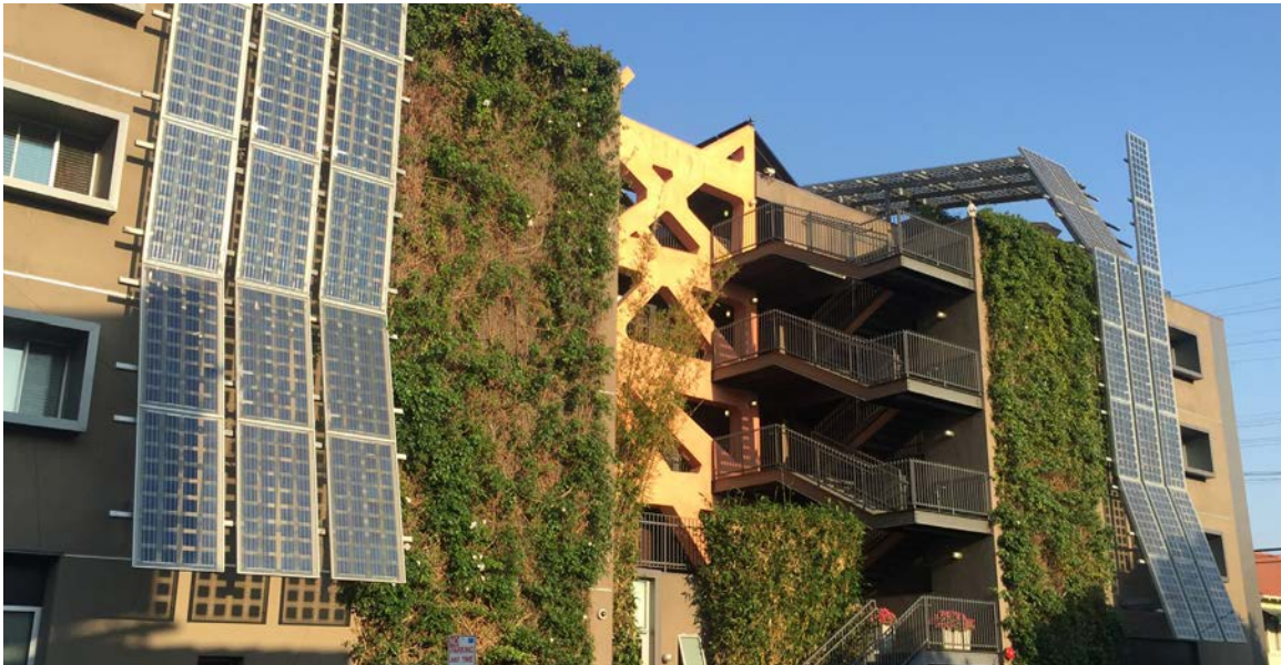
Buildings like the Sierra Bonita Apartments have reduced utility costs for tenants by installing solar arrays on the roof and side wall of the building.
