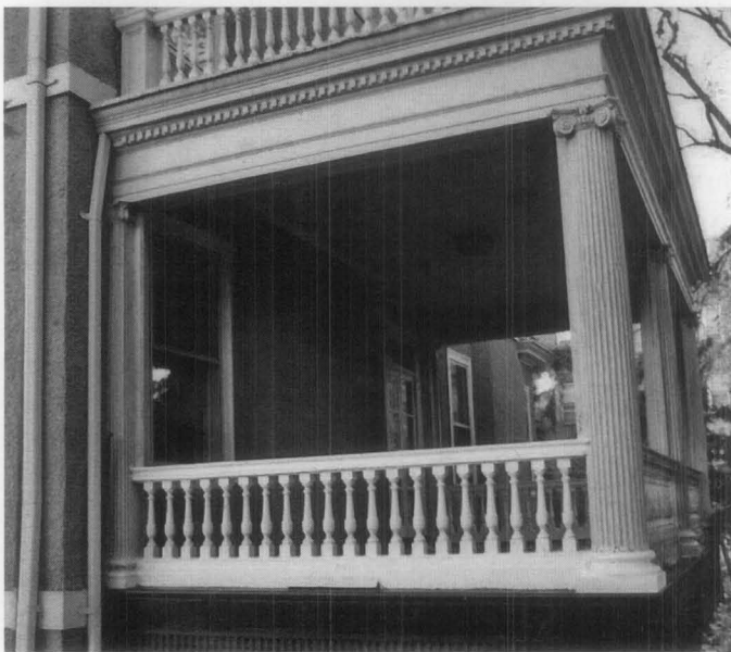
Figure 17. The porch's structural system must be capable of supporting today's loads. In this case moisture led to the deterioration of the wood girder at the corner, creating a major structural deficiency (top). A new solid timber was installed to replace the girder (middle); alternatively a built-up girder could have been used since a fascia board would conceal it. The column base was repaired and portions replaced and the balustrade and column reset and secured (bottom). Photos: Paul Marlowe, Marlowe Restorations.
