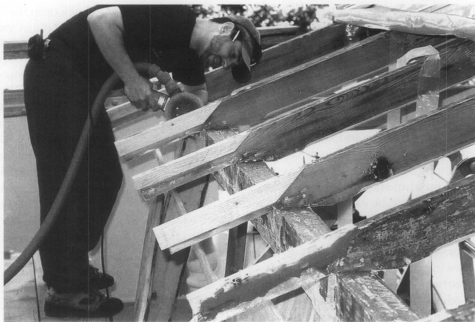
Figure 9. The ends of porch roof rafters are often susceptible to moisture decay. When concealed by a soffit or ceiling, rafters can be repaired by adding new sister boards. Where roof rafter ends are exposed, splicing new wood onto the old (dutchman repair) and use of epoxy consolidants and fillers both preserve sound historic fabric while retaining the historic appearance. Photo: Paul Marlowe, Marlowe Restorations.
