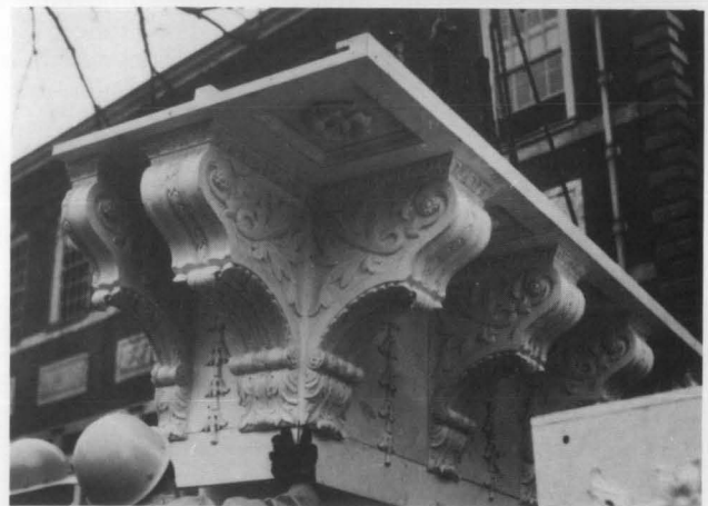
A fiberglass cornice for the reconstruction of an 18th-century wooden clockcase is being lifted in pre-fabricated sections. The level of detail is intricate and of high quality. Photo: Courtesy of Independence National Historical Park.
