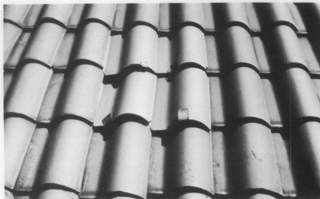
Repairs on this pantile roof were made with new tiles held in place with metal hangers. (Main Building, Ellis Island, New York)
