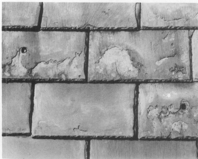
This detail shows slate delamination caused by a combination of weathering and pollution. In addition, the slates have eroded around the repair nails, incorrectly placed in the exposed surface of the slates. (Lower Pontalba Building, New Orleans, photo courtesy of Building Conservation Technology, Inc.)
