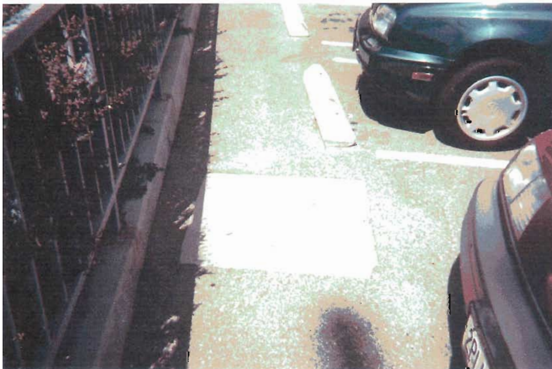
Abandoned Well in Former Gas Station
