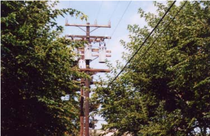
Utility wires over south lawn.
